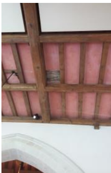
Plaster fall from North Aisle
